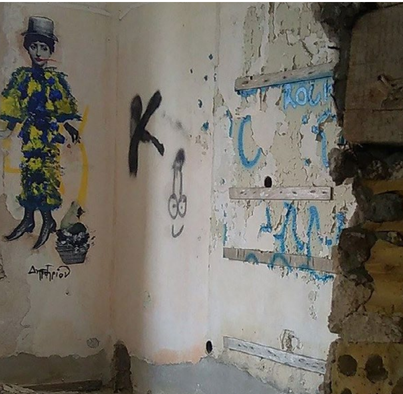
Figure 3. The lady and the cat. Are those broken windows from weathering storms, or from careless and thoughtless human beings? I see you, dear house. You are empty, but not forgotten. Photograph ©Anna Dimitriou
