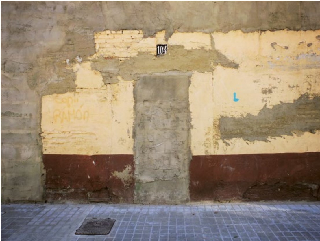
Figure 6. The owner has blocked the doors, windows and air vents with heavy layers of cement.
