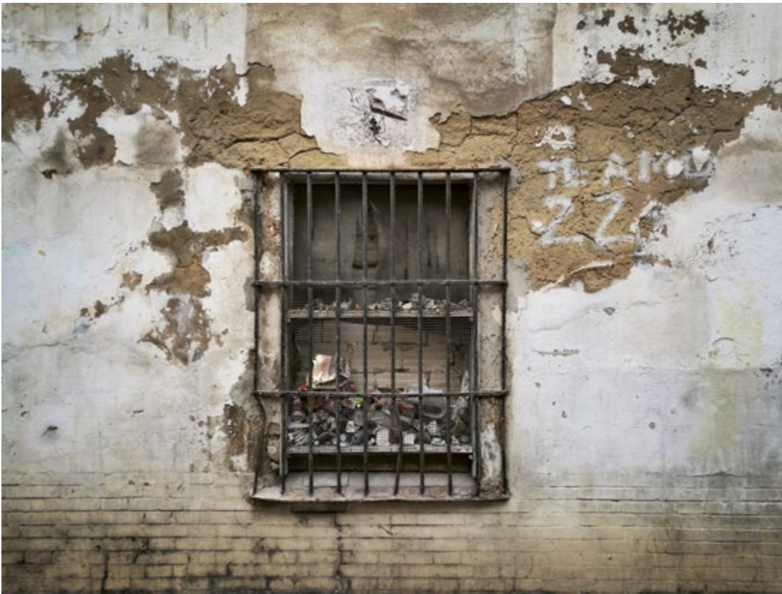
Figure 5. Abandoned house. The window is sealed with bricks from the inside. On the wall, someone has written: Te amo , 'I love you', in white paint. Sixty percent of the houses in the area are over 50 years old, and during the last twenty years around 200 houses have been demolished (Hervás Más, 2017).
