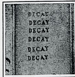
Decay is written on door of Queensboro Bridge
